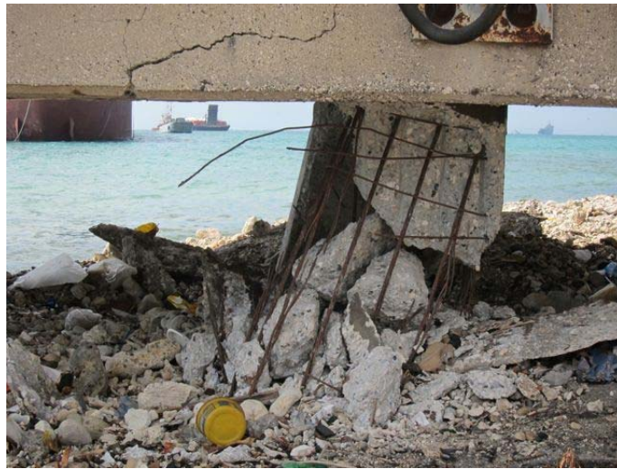
Figure 6.16: (top) Damage to piles supporting the pedestrian bridge connecting the South Pier to the island (photo taken facing South) and (bottom) extensive damage to the landward row of piles (photo taken facing West) (N18.554628, W72.351492)
