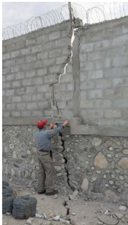
Figure 6.23 Lateral spreading in the storage yards in the northern part of the port facility. Lateral spread crack passes through a stone/masonry wall. Photo taken facing South. (Approximate long. and lat. of photo: 18^{\circ}33'35.15''\text{N} 72^{\circ}20'56.18''\text{W} )
