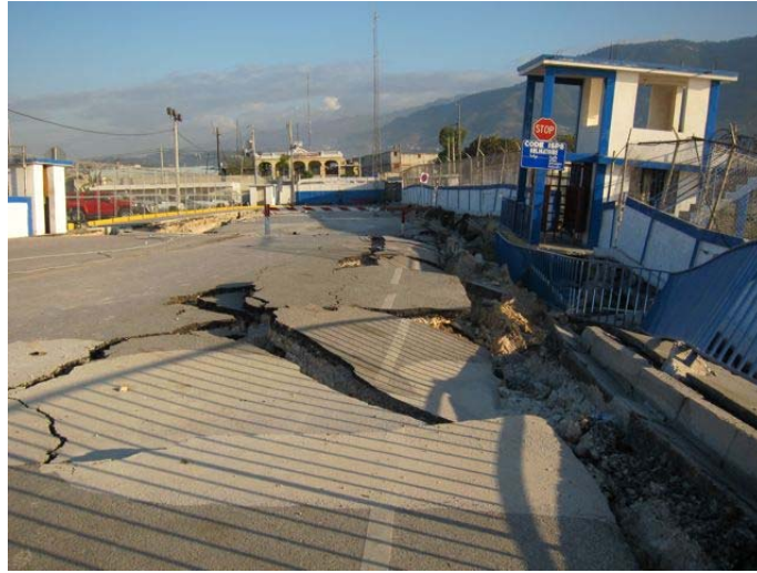
Figure 6.25: Damage to entrance road caused by lateral spreading. Photo taken facing South-East. (Approximate long. and lat. of photo: 18°33'11.61"N 72°20'52.50"W)
