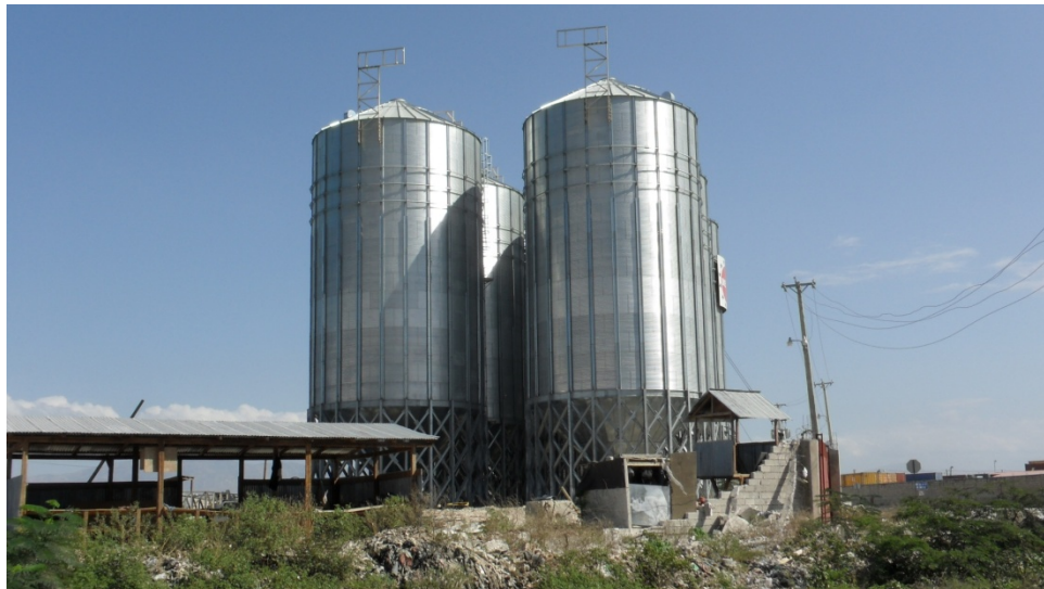
Figure 6.19 Post-earthquake photo of steel grain hopper silos (photo taken facing North). The silos showed no visible signs of distress. (N18.558431, W72.350350)
