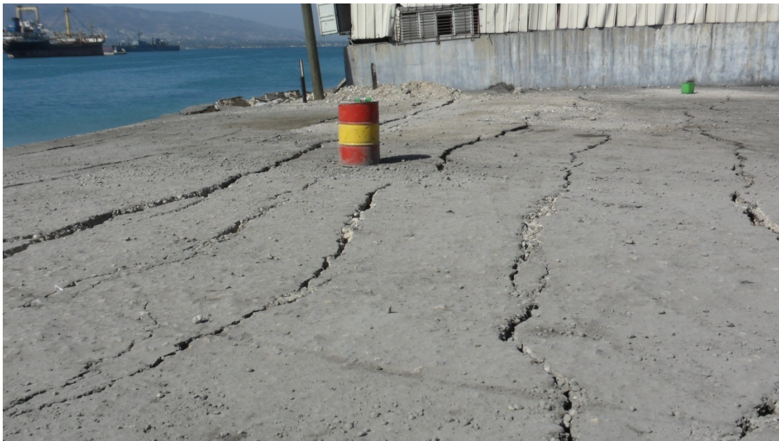
Figure 6.7 Lateral spreading between the two metal warehouses, adjacent to the collapsed North wharf (left). A cumulative total of 89 cm of horizontal movement (determined by crack width) was measured in a zone extending inland approximately 30 m from the post-earthquake shoreline. Post-earthquake imagery indicates lateral spread cracking extended 50 m inland. (N18.556696, W72.34787)
