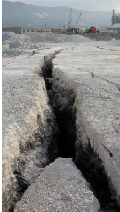
Figure 6.22 Lateral spreading in the storage yards in the northern part of the port facility. Photo taken facing South. ( 18^{\circ}33'41.76''\text{N} 72^{\circ}20'52.25''\text{W} )
