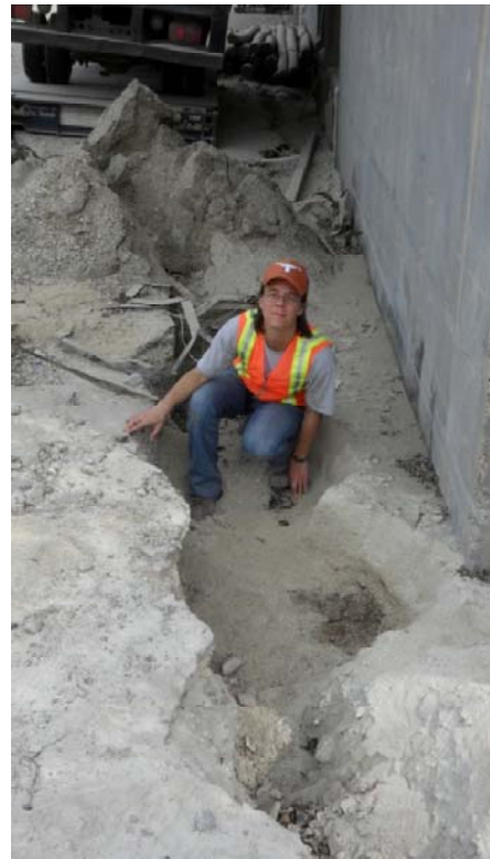
Figure 6.10 Liquefaction and lateral spreading adjacent to the north side of the metal warehouses. Photo on top taken facing west, photo on bottom taken facing east. (N18.556961, W72.349751)
