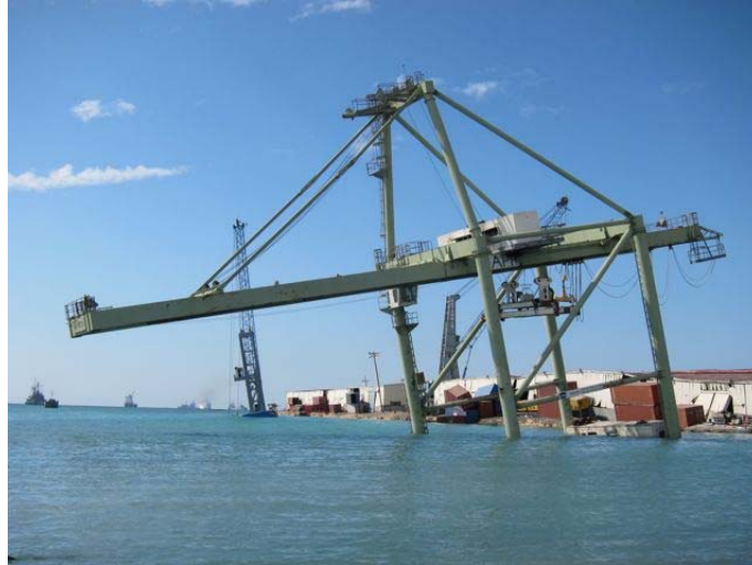
Figure 6.12 Submerged 15-m gauge container crane (foreground) and mobile crane (background). Photo taken facing west. (N18.55598, W72.348564)
