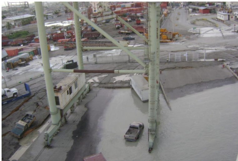
Figure 6.13 Photo taken immediately after the earthquake with the crane in its most eastward position and with the landside legs of the crane above water. Photo taken facing east. Source: unknown (N 18.556056, W72.347981)
