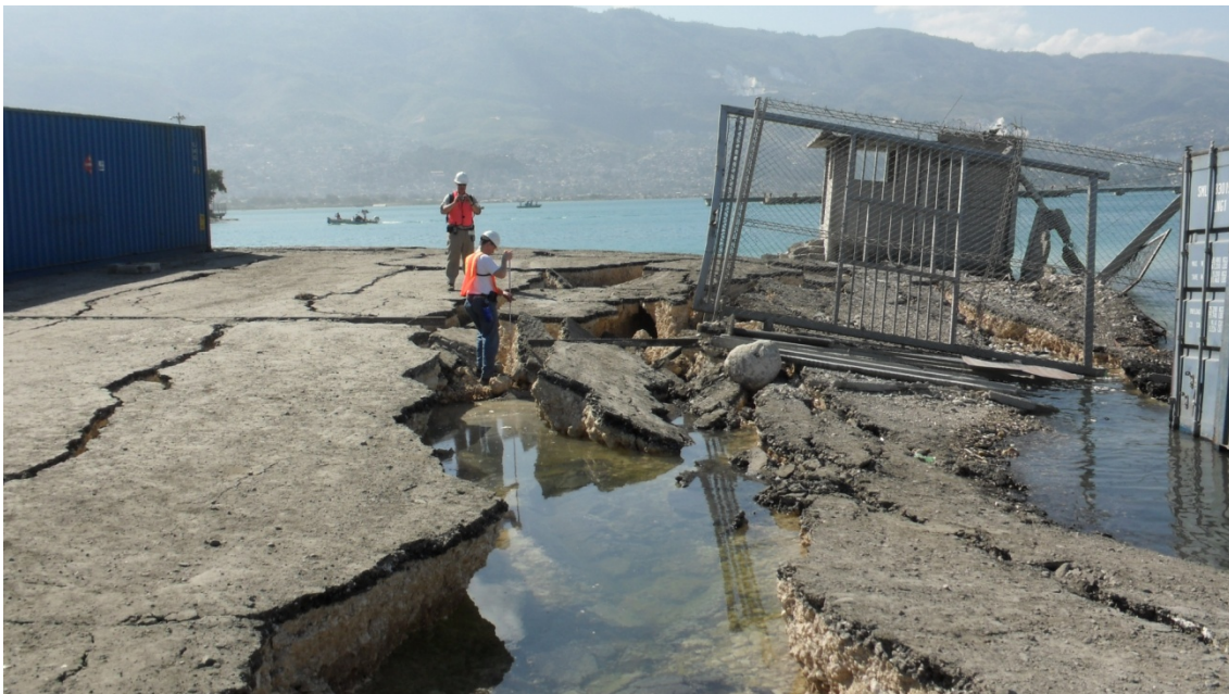
Figure 6.9 Lateral spreading west of the two metal warehouses. Photo taken facing south with the metal warehouses to the left. (N18.557075, W72.352045)
