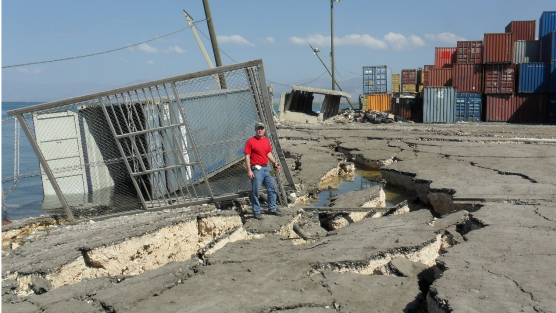
Figure 6.8 Lateral spreading west of the two metal warehouses. Photo taken facing north with the metal warehouses to the right. (N18.557075, W72.352045)
