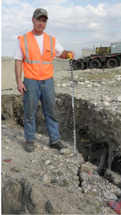
Figure 6.24 Lateral spreading in the storage yards in the northern part of the port facility. A unique feature of this lateral spread is that the fill is garbage. However, it is believed that the liquefaction of the sand below garbage is the cause of the lateral spreading. Photo taken facing North-East. (Approximate long. and lat. of photo: 18^{\circ}33'38.93''\text{N} 72^{\circ}20'54.89''\text{W} )
