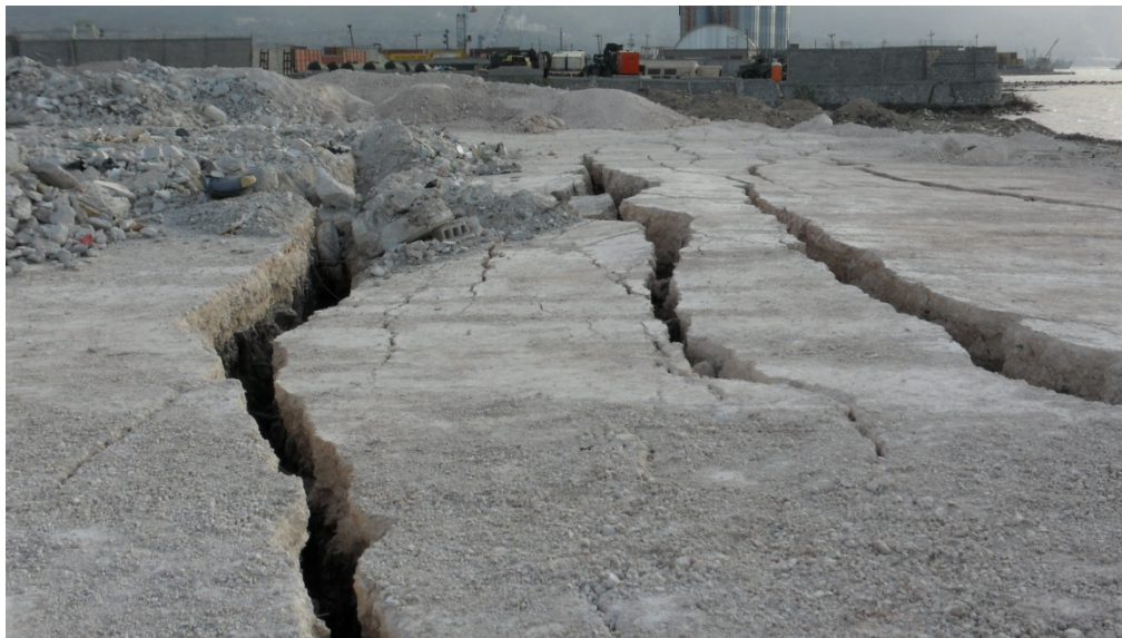
Figure 6.21 Lateral spreading in the storage yards in the northern part of the port facility. Photo taken facing South. ( 18^{\circ}33'41.39''\text{N} 72^{\circ}20'52.51''\text{W} )
